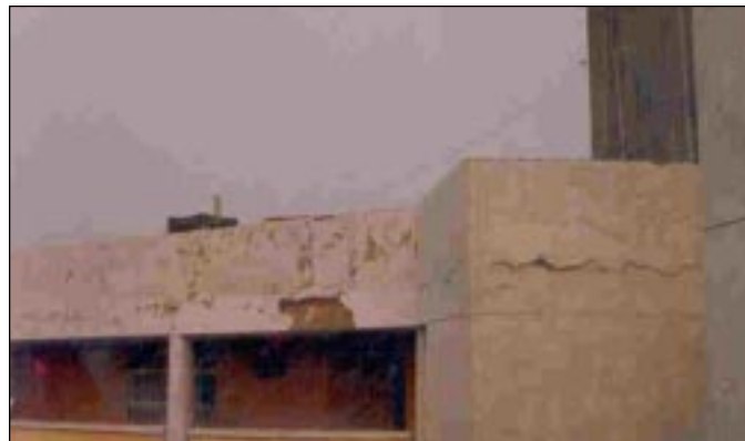
Plate 6: Spalled concrete in RCC parapets →
