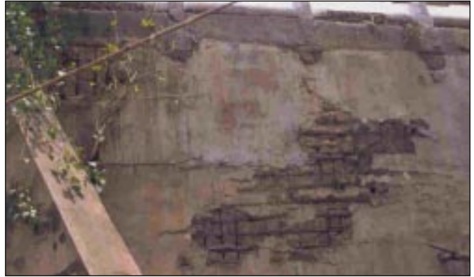
Plate 2: Typical damage of the Counter-fort Retaining Wall →
