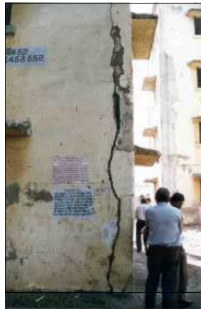
Plate 7: Cracked RCC Column at corner due to Corrosion of steel reinforcement →
