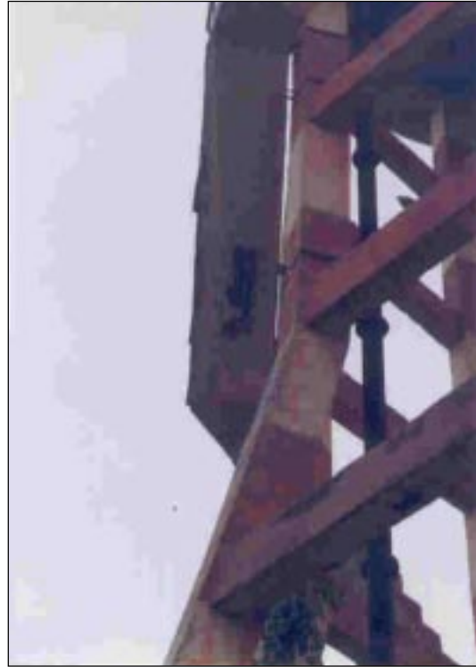
Plate 2: Spalled cover concrete and cracks in waist slab and bracing beams.
