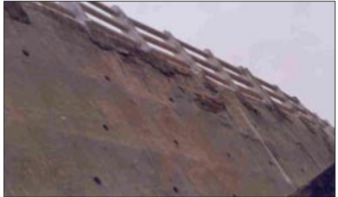
Plate 3: Typical damage of the Counter-for Retaining Wall →
