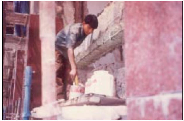
Plate 13: Passivating and Bond Coat Applied over Prepared Surface of steel and concrete in a Beam →
