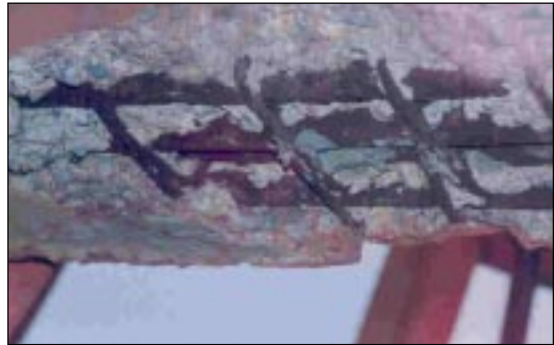
Plate 4: Spalled and honey combed cover concrete and congested bottom reinforcement of bracing beam.
