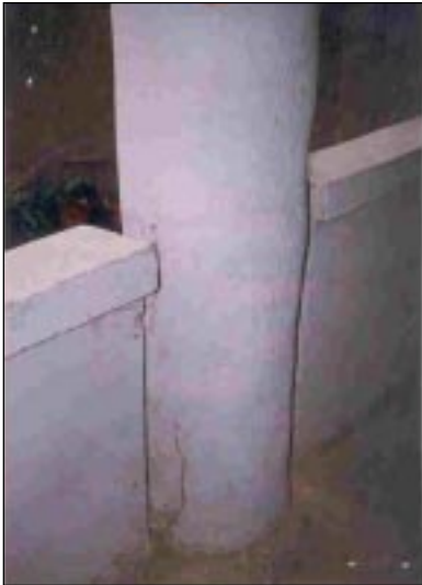
← Plate 2: Cracks in column earlier repaired by guniting
