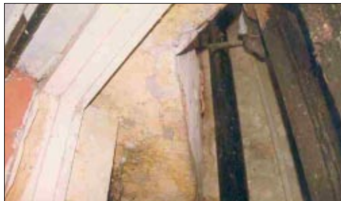
Plate 8: Inaccessible and inadequately sized Service Shafts →
