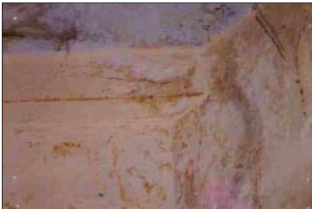
← Plate 4: Signs of leakage and seepage
