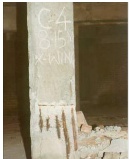
Plate 4: Rust Signs in RCC column →
