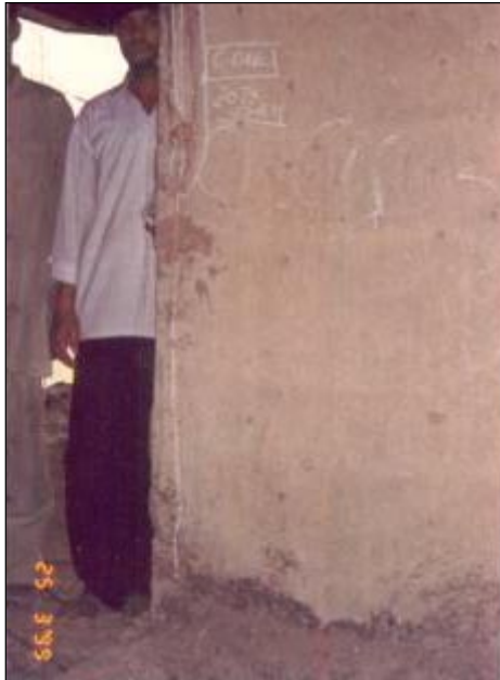
← Plate 3: Corrosion cracked column
