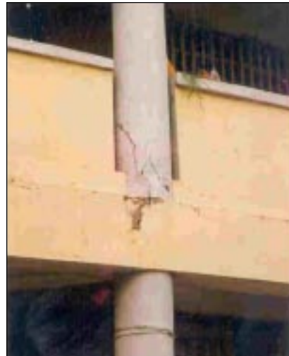
Plate 3: Crushed cover concrete and cracking along main reinforcement →
