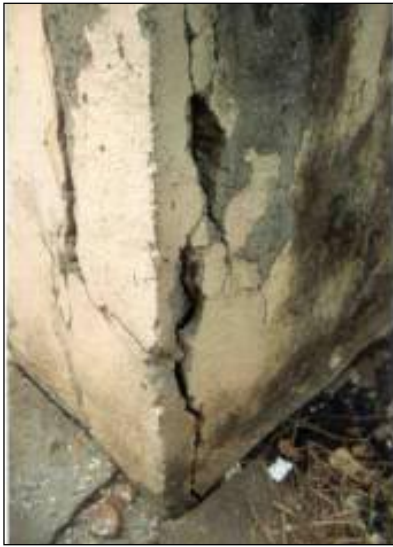
← Plate 6: Cracked RCC column near plinth protection
