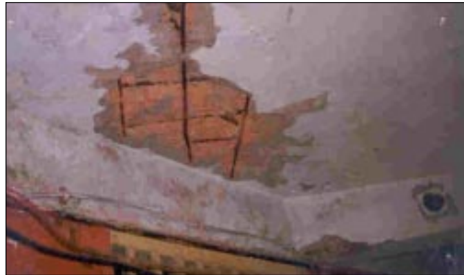
Plate 5: Spalled cover concrete in RCC slab →
