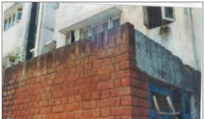
Plate 8: Horizontal cracks in Masonry Walls of Single storeyed Garages →
