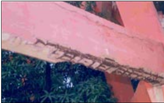
Plate 3: Spalled cover concrete and exposed corroded reinforcement of beam. Longitudinal crack in the top cover concrete.
