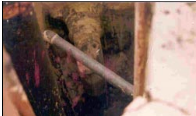
Plate 7: Broken & missing rainwater pipe →
