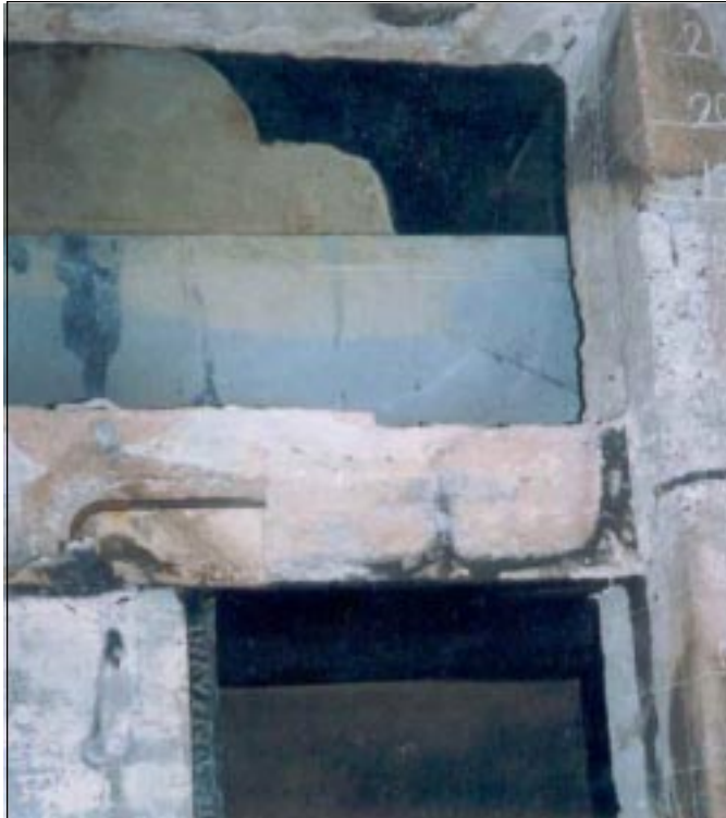
Plate 1: Damaged Column & Beam Junction
