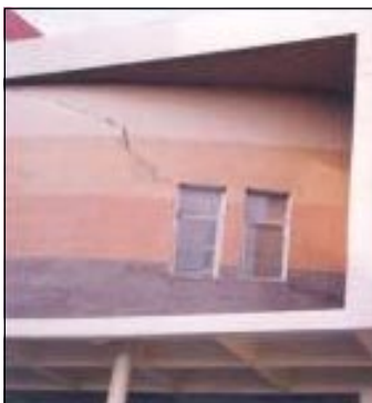
← Plate 4: Cracks in curved wall resting on circular beam
